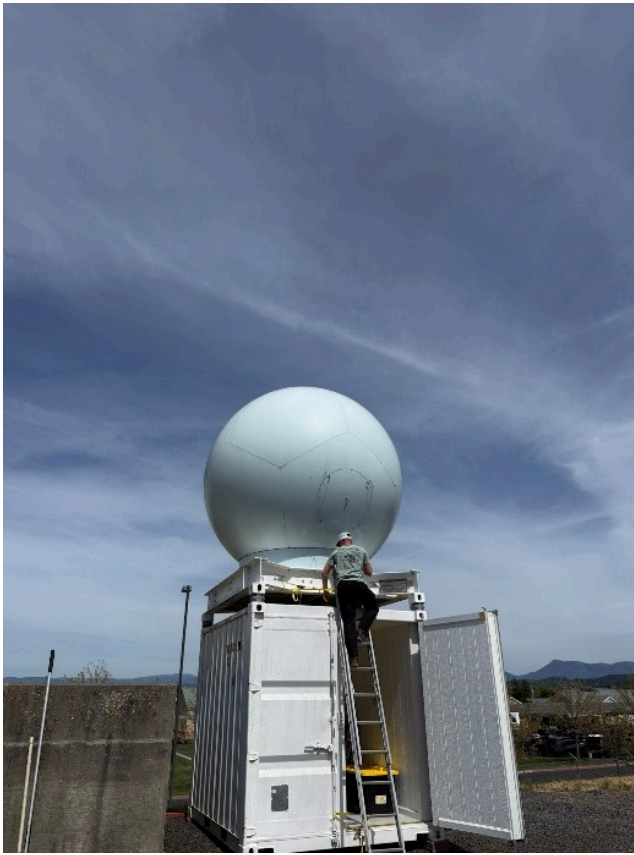
Sonoma Water Engineer II Erik Paulson replaces the access hatch of the X-Band Radome at the Airport Treatment Plant
